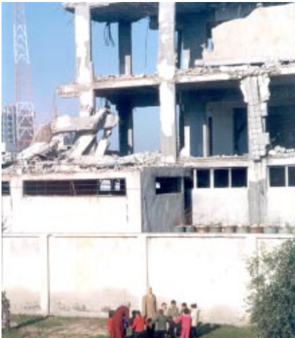
An air raid on a Palestinian police base next to the al-Nour Rehabilitation Centre for the Visually Impaired caused heavy damage to the Centre in the spring of 2002. The Centre has been repaired and the children have been able to return to class but the surrounding buildings still loom precariously over the RCVI school yard. UNRWA runs a regular program of elementary education at the Centre plus special programs for visually impaired children and an outreach program throughout the Gaza Strip. It is a school for children with special needs but they, too, have the right to education. The air raid, the damage and ensuing emotional trauma is typical for thousands of other students in the West Bank and Gaza Strip. Photo: Ron Wilkinson.
